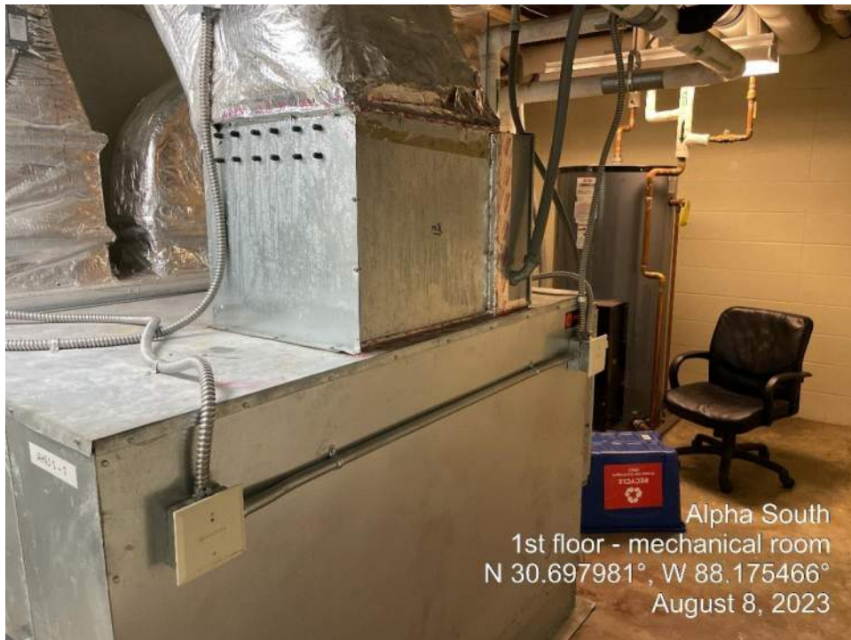
Photograph 18 – Alpha South – 1 st Floor Mechanical Room.
