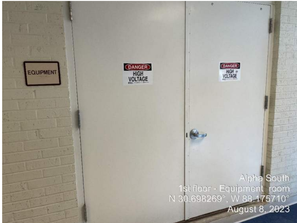
Photograph 19 – Alpha South – Electrical Equipment Room.
